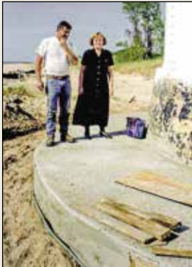
Mary James and "Willie" from Carr Creek Construction inspect the new sidewalk, 1998
