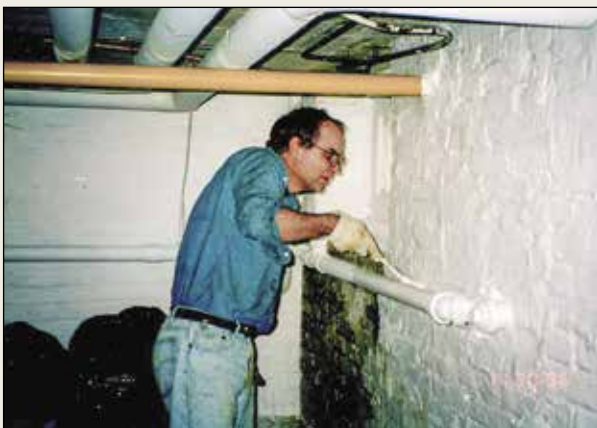
Bob Sperling doing maintenance in the basement at BSP, 1996
