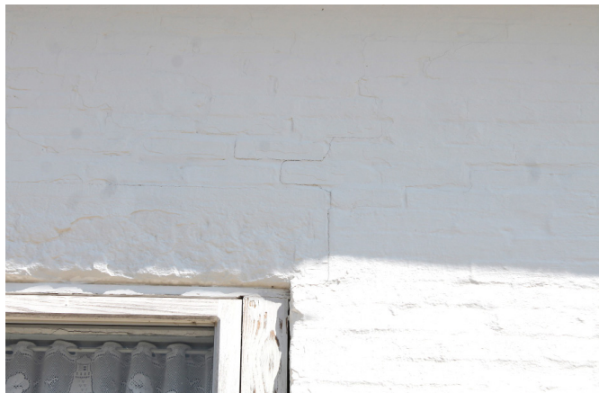
Figure 1D-76 Step cracking along edge of stone masonry lintel at the western end of the south facade.
