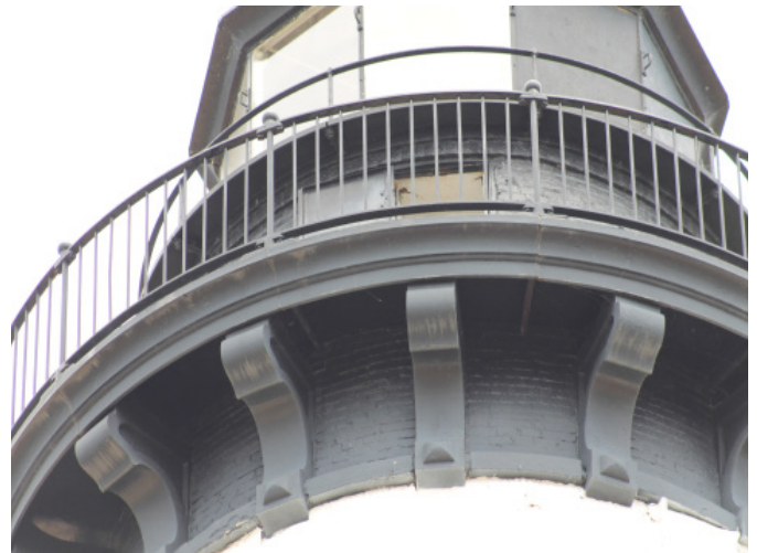
Figure 1D-276 Rail posts do not align with brackets below lantern balcony floor level.
