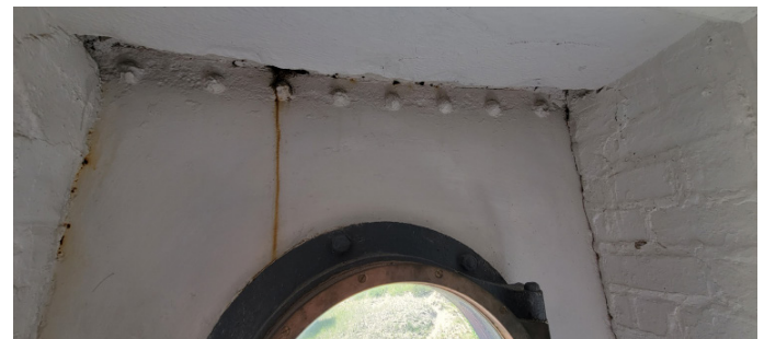
Figure 1D-250 Corrosion staining at window well at watch room floor level; note steel is tight to the brick masonry (no cementitious fill between the masonry and the steel plate this level).
