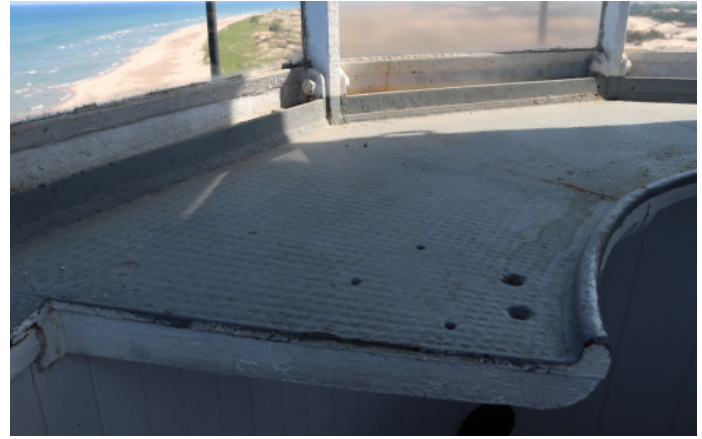
Figure 1D-320 Cast iron floor in the Lantern and base of Lantern windows.
