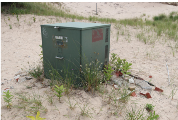
Figure 1D-239 Electric transformer located off the southwest corner of the Keepers' Dwelling.
