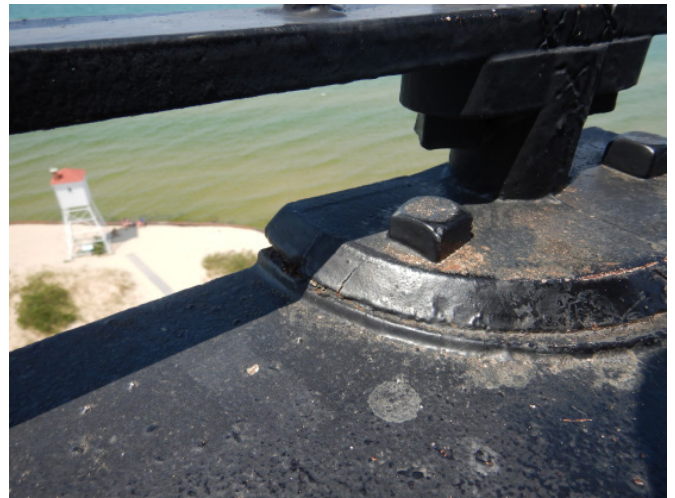
Figure 1D-275 Cracked base plate at bolt location at rail post at exterior balcony at lantern level.
