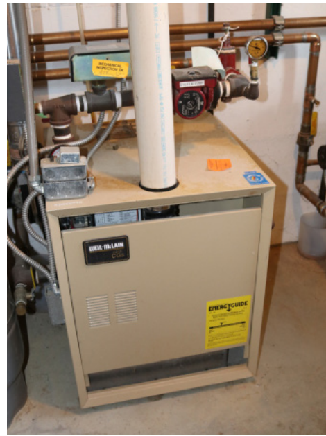
Figure 1D-205 Weil-McLain 167,000 btuh propane gas fired boiler.
