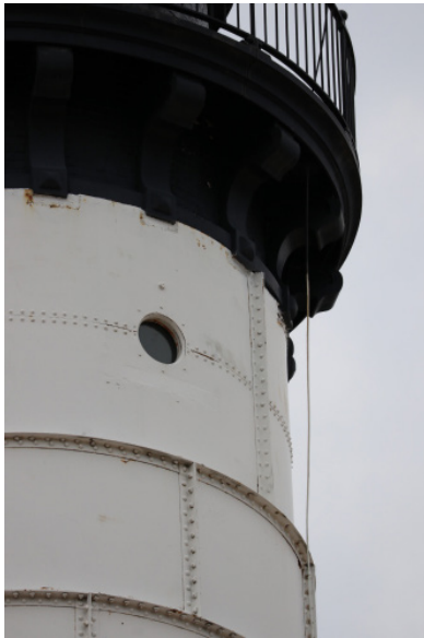
Figure 1D-281 “Porthole” style window in the metal cladding surface of the Light Tower.
