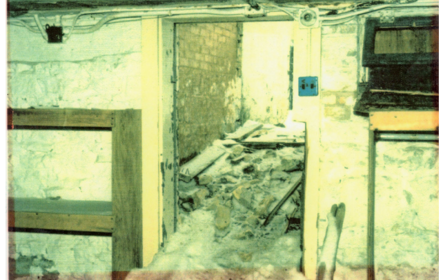
Figure 1B-80: Undated photo showing debris at the basement stair to the exterior.
