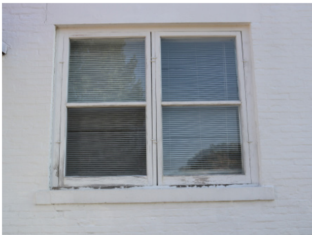
Figure 1D-102 Exterior view of first floor Living Room double hung windows and storm sash on the south elevation.
