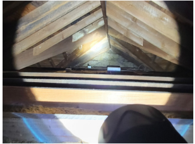
Figure 1D-59 Roof framing at ridge of east half of Keepers' Dwelling; note single nominal 2x members at dormer framing each side.
