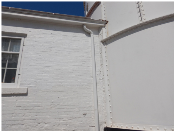
Figure 1D-224 Cracking present at north end of east wall at intersection of tower.
