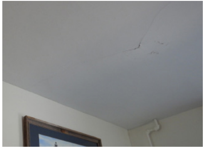
Figure 1D-55 Cracking in ceiling near center of room and extending up from corner of door.
