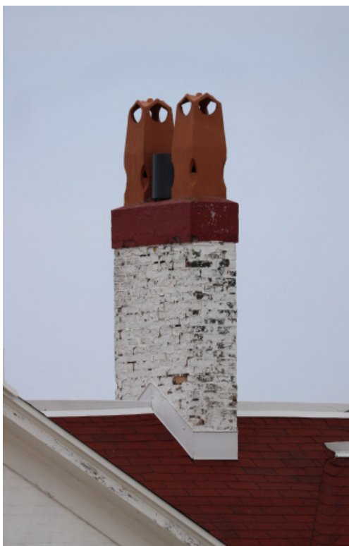
Figure 1D-90 Deteriorated brick and paint on the brick masonry chimney.
