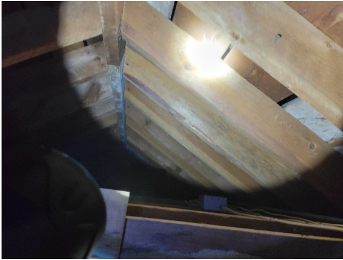
Figure 1D-58 Roof framing at ridge of west half of Keepers' Dwelling; note skip-board 1x sheathing.
