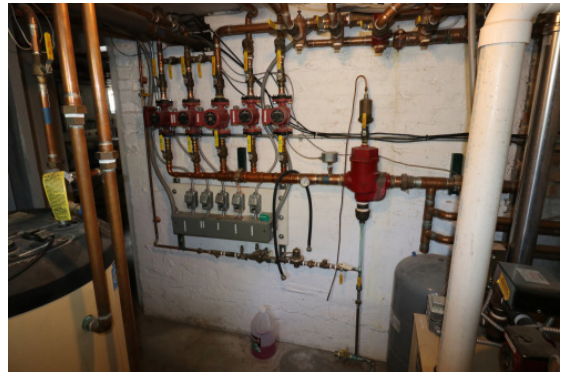
Figure 1D-206 Heating system zone control valves in the Basement Mechanical Room.
