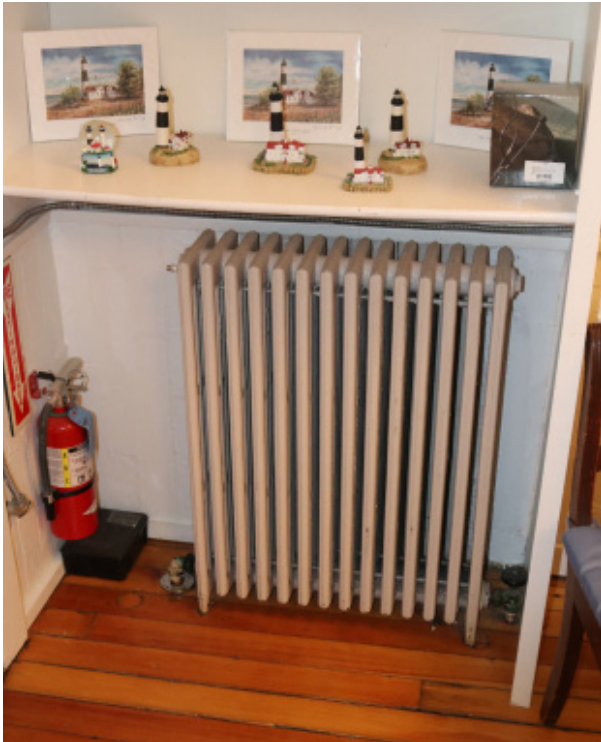
Figure 1D-208 Typical cast iron radiator. This one is located in the Gift Shop (former Kitchen).
