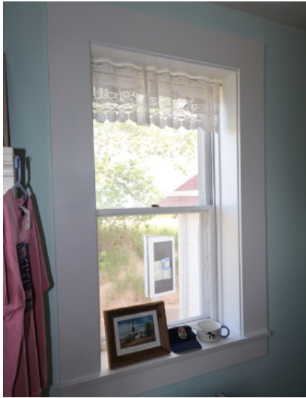
Figure 1D-104 First floor double hung window in the west part of the Keepers' Dwelling.
