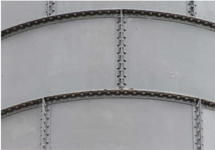
Figure 1D-268 Vertical angles deformed at ends likely due to "rust jacking" forces separating the angle sections.
