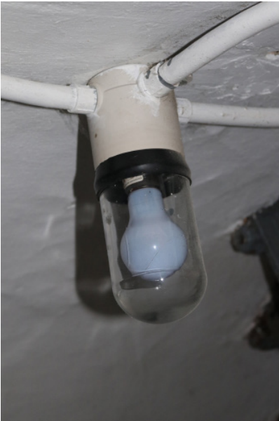
Figure 1D-330 Interior light fixture at the bottom level of the Light Tower.
