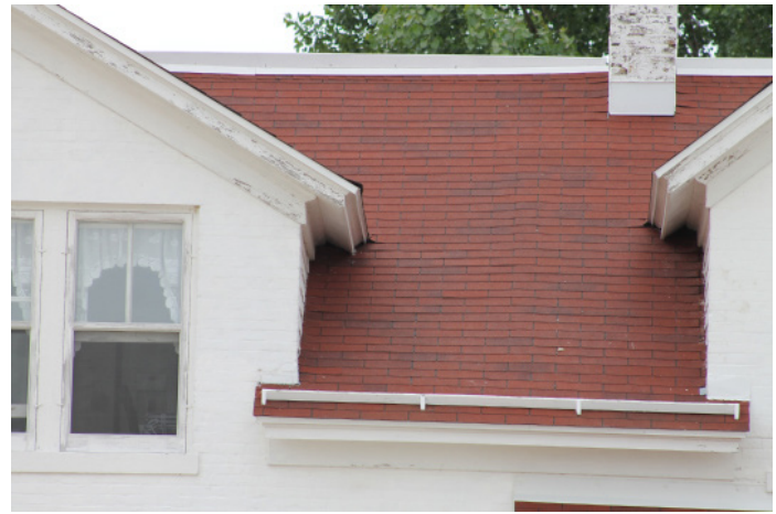
Figure 1D-63 Sloping of roof adjacent to center masonry demising wall at chimney on eastern portion of the Keepers' Dwelling.
