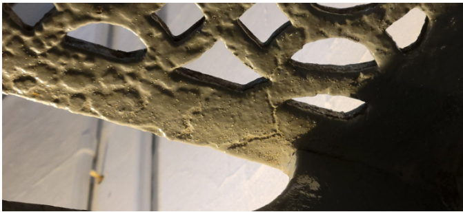
Figure 1D-257 Pitting of and potential cracking through the coated cast iron lattice stair tread.
