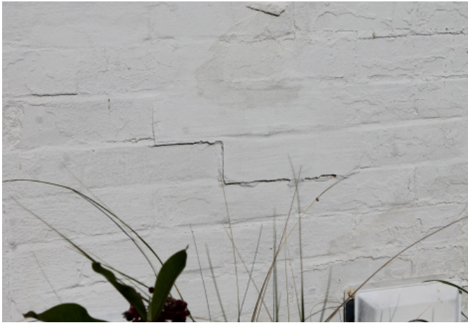
Figure 1D-74 Step cracking on east facade, north of basement windows.
