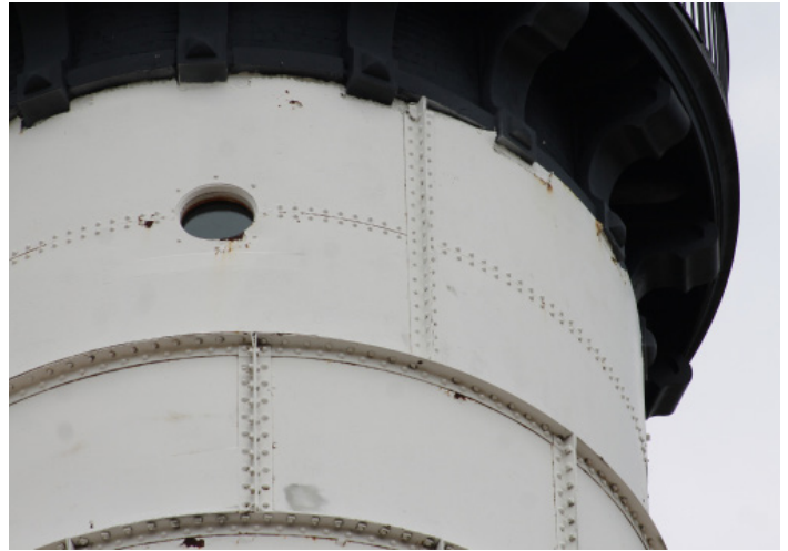
Figure 1D-271 Fastener misalignment in horizontal leg where upper cladding meets lower cladding around perimeter of tower.
