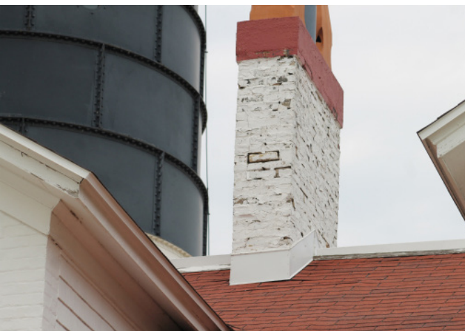
Figure 1D-73 Mortar around brick in chimney missing.
