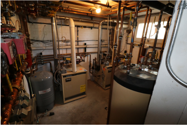
Figure 1D-202 Propane fired boilers for building heat and domestic hot water located in the Basement Mechanical Room.
