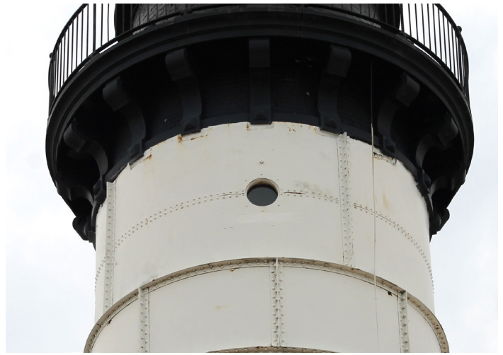
Figure 1D-270 Corrosion and potential displacement present at lantern balcony bracket locations at top of upper level metal cladding.
