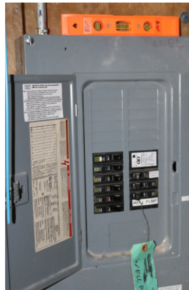
Figure 1D-211 Electric sub-panel located in the Basement.
