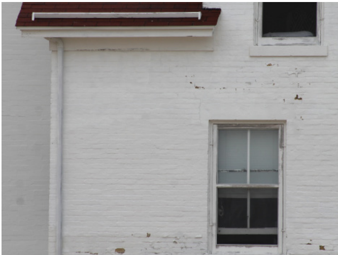
Figure 1D-75 Cracking extending between eastern corner of window and roof level at north facade.
