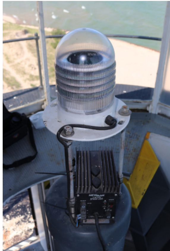
Figure 1D-332 "SeaLite" LED navigation light in the Lantern.
