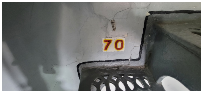
Figure 1D-247 Cracking in plaster at stair tread.
