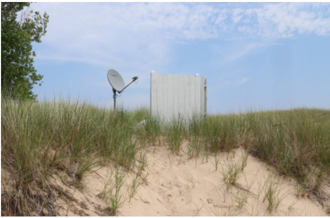
Figure 1D-17 Satellite dish and fenced enclosure.
