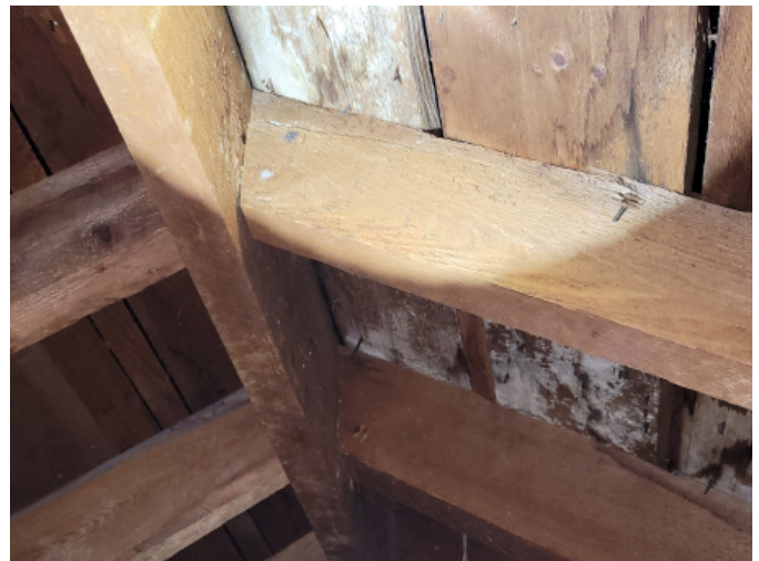
Figure 1D-60 Difference of color in skip-board sheathing at west half of roof; rafters are tight to ridge board.
