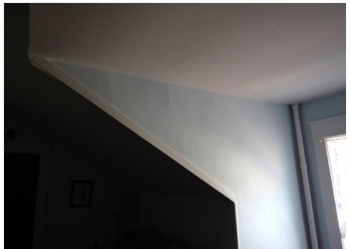
Figure 1D-53 Cracking in west wall of north dormer at second floor living area.
