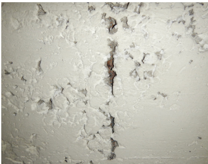
Figure 1D-51 Steel reinforcing visible where concrete was poorly consolidated during original construction.
