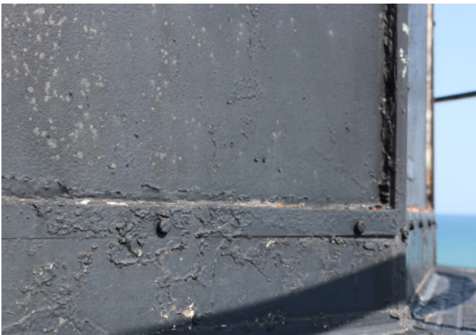
Figure 1D-306 Base of Lantern with deteriorated paint finish.
