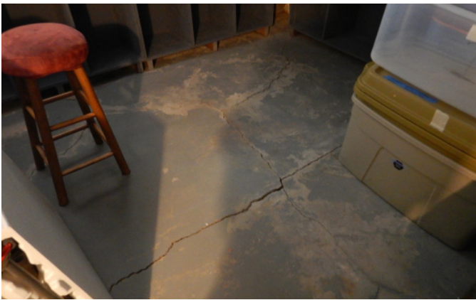
Figure 1D-38 Cracked and heaved slab on ground in southwest quadrant of basement of keepers dwelling
