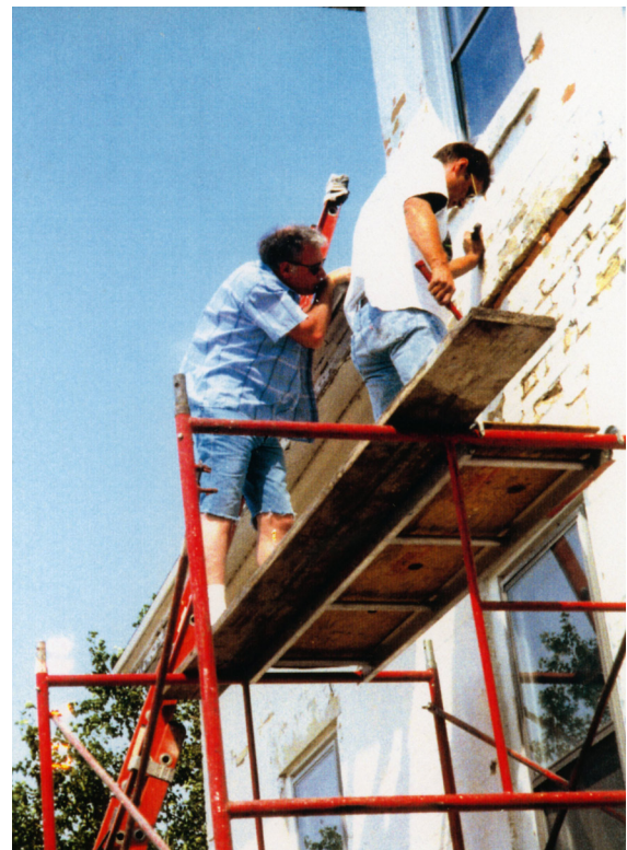
Figure 1B-96: Circa 1990s photo of SPLKA volunteers repointing the masonry wall of the Keepers' Dwelling.
