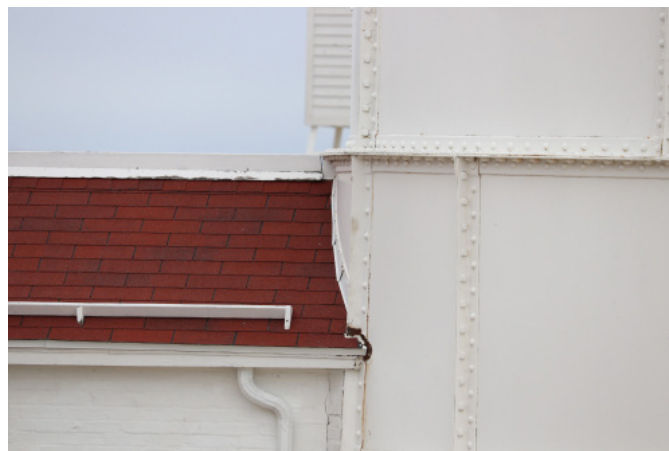
Figure 1D-230 Metal step flashing at the intersection of the asphalt shingle roof with the metal walls of the Light Tower.
