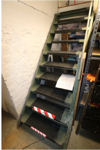
Figure 1D-177 Central stair from the first floor to the east part of the Basement.
