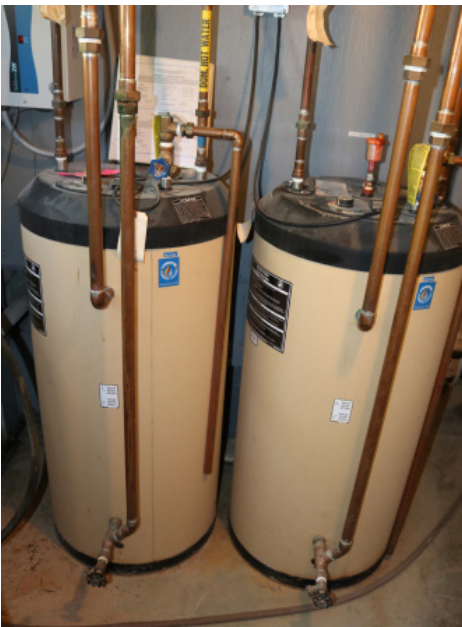
Figure 1D-204 Indirect fired hot water heaters for domestic hot water located in the Basement Mechanical Room.
