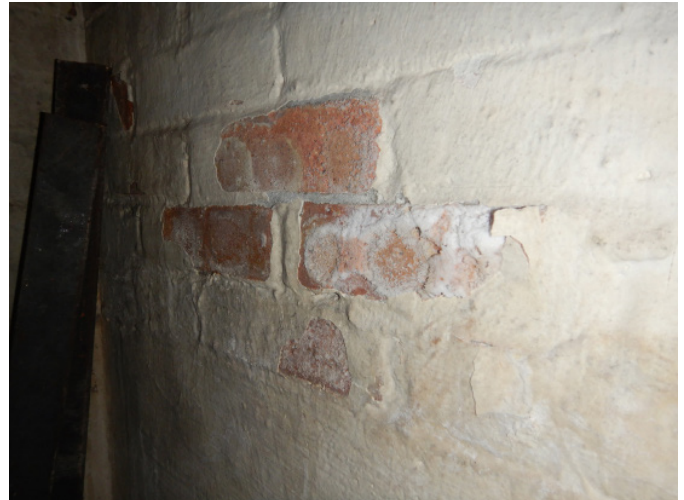
Figure 1D-42 Missing and peeling coating, efflorescence present on south brick masonry foundation wall.
