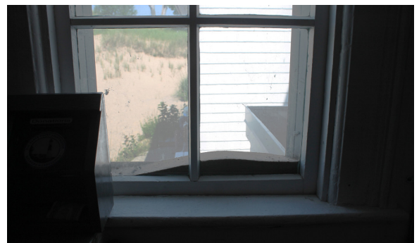
Figure 1D-227 Sand accumulation on sill of east window.
