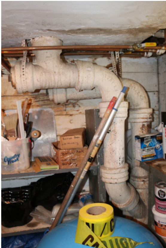
Figure 1D-198 Cast iron sanitary piping in the Basement.
