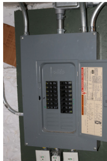
Figure 1D-212 Electric sub-panel located in the Basement.
