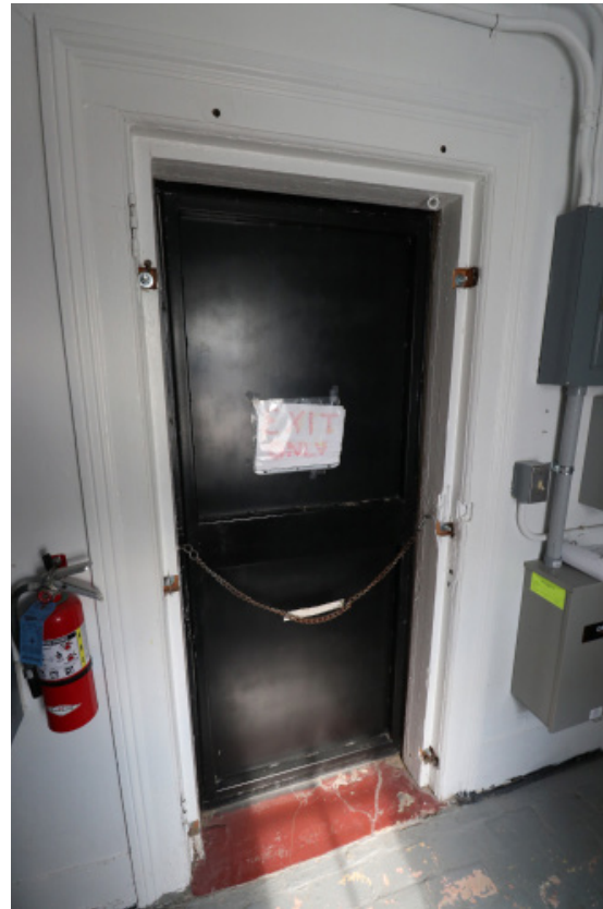
Figure 1D-235 Interior view of the steel plate door and hardware remnants.
