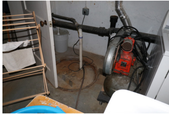
Figure 1D-200 Basement sump pump located near the southeast corner.
