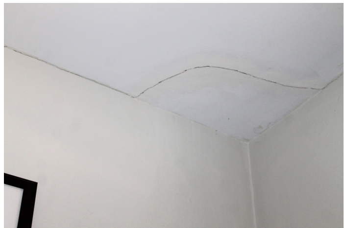
Figure 1D-57 Cracking reoccurred after previous repair attempt.
