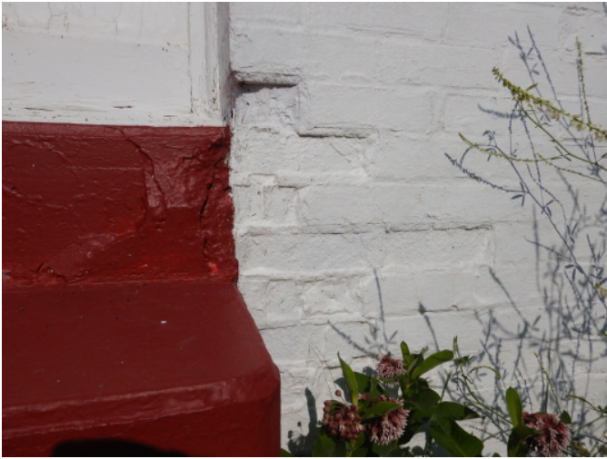
Figure 1D-69 Coating applied over spalled brick.
