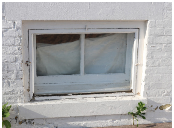
Figure 1D-99 Basement window and deteriorated storm sash on the south elevation.
