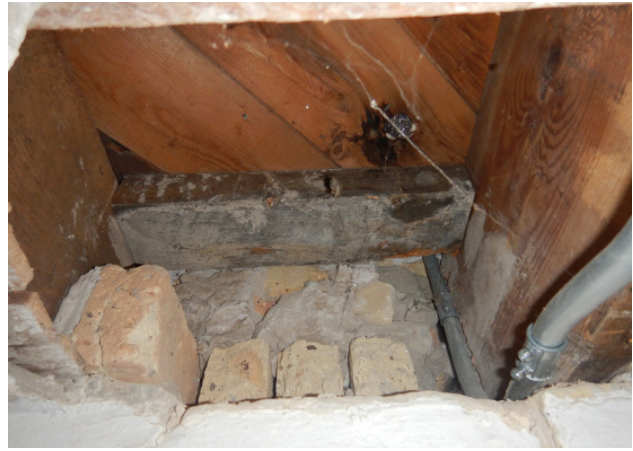
Figure 1D-46 Floor joists bearing at south brick basement wall; note diagonal subfloor and wood blocking between joists.
