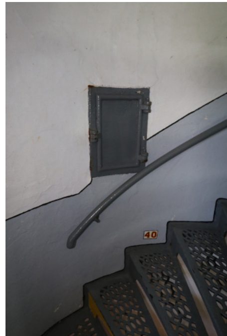
Figure 1D-311 Metal door for access into a wall cavity. Metal stair handrail is also seen.
