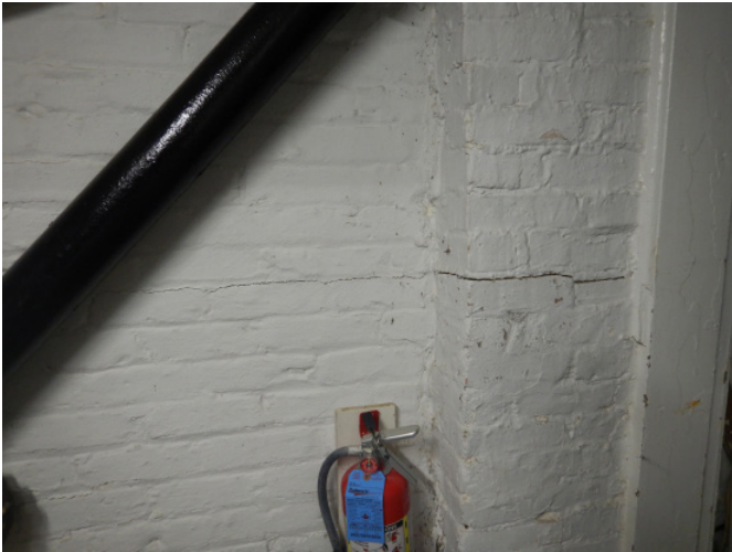
Figure 1D-43 Horizontal crack in south brick masonry foundation wall.
