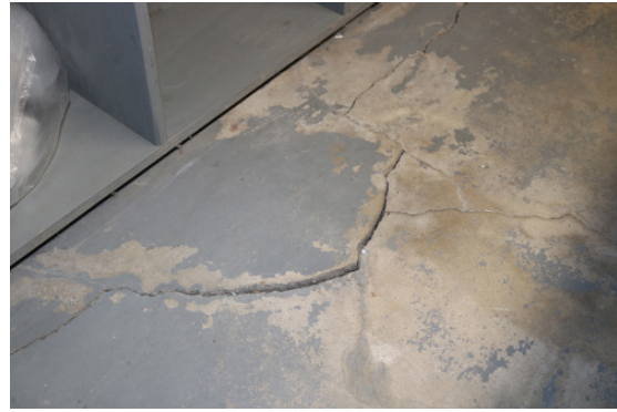
Figure 1D-191 Concrete floor slab cracking in the west part of the Basement.
