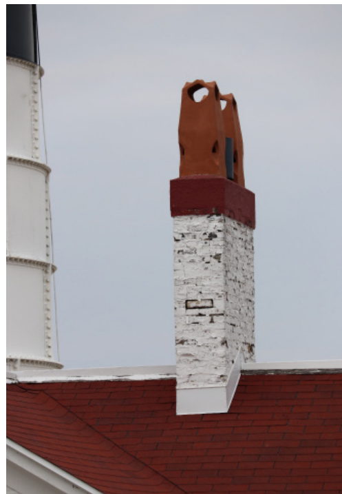
Figure 1D-89 Deteriorated brick and paint on the brick masonry chimney.
