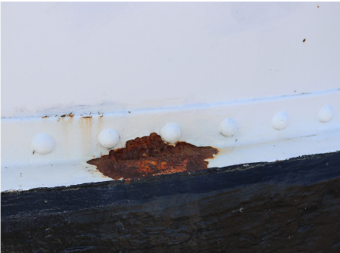
Figure 1D-278 Deteriorated paint finish and corrosion of steel.
