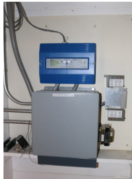
Figure 1D-207 Boiler control unit in the Basement Mechanical Room.
