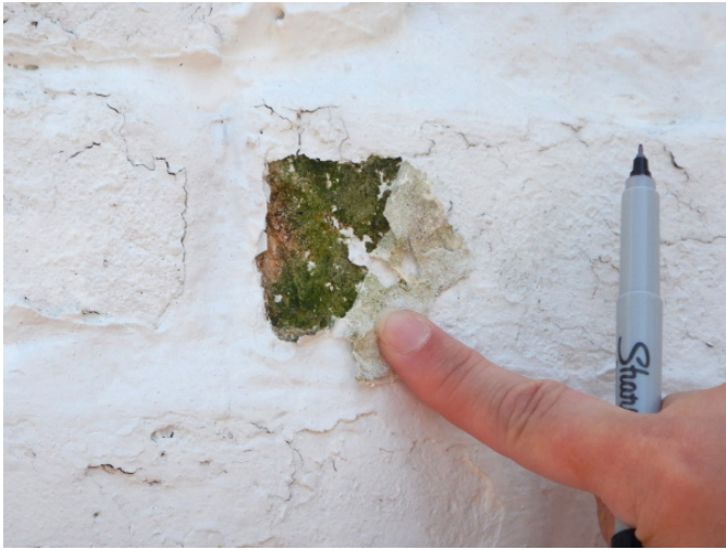
Figure 1D-64 Organic growth located between the brick masonry exterior face and the exterior coating.
