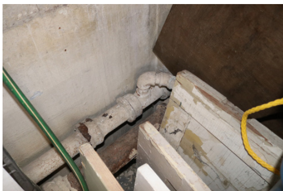
Figure 1D-199 Cast iron sanitary piping exiting the southeast corner of the Basement.
