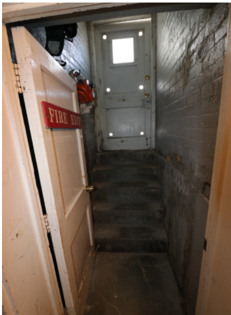
Figure 1D-178 Concrete stair from the Basement to the exterior on the north elevation.
