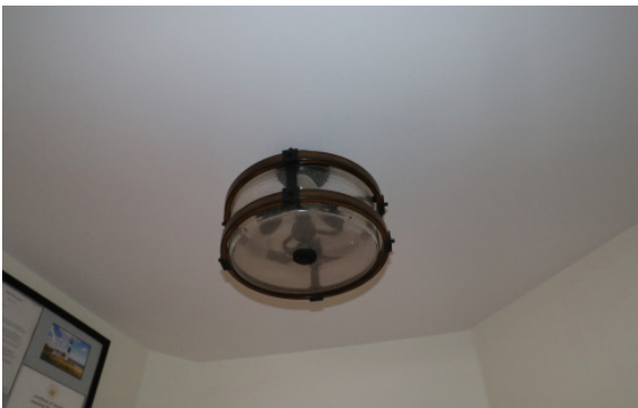
Figure 1D-216 Interior light fixture example.
