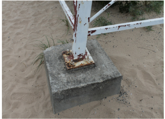
Figure 1D-338 Northwest concrete foundation, top of corner is spalled.
