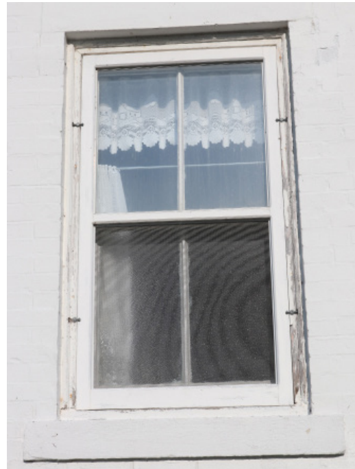
Figure 1D-101 Exterior view of first floor Bathroom double hung window and storm sash on the east elevation.
