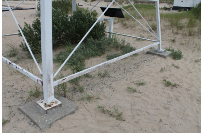
Figure 1D-337 Southern concrete foundations; note corner is spalled from southwest (left) foundation.
