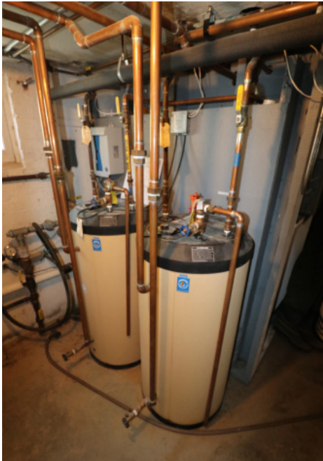
Figure 1D-203 Indirect fired hot water heaters for domestic hot water located in the Basement Mechanical Room.
