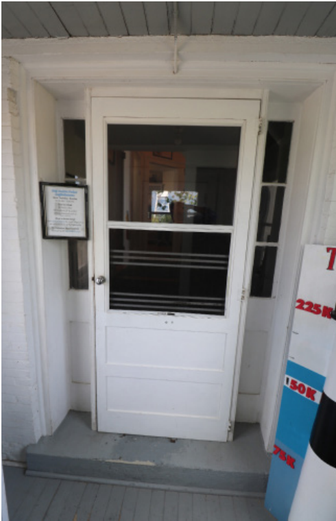
Figure 1D-114 Wood storm door at the Gift Shop entry from the West Porch.
