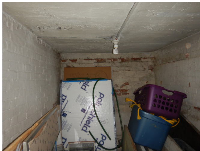
Figure 1D-50 Underside of concrete slab at southeast corner vestibule above; note condition of brick on east and south exterior walls of this basement level storage room.
