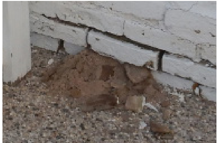
Figure 1D-78 Sand obtained from behind the loose brick when brick was removed.
