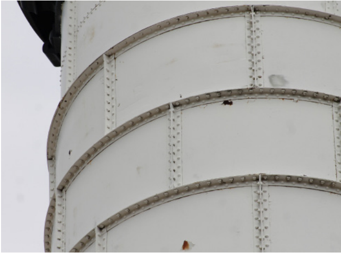
Figure 1D-273 Fastener misalignment in horizontal leg where upper cladding meets lower cladding around perimeter of tower.
