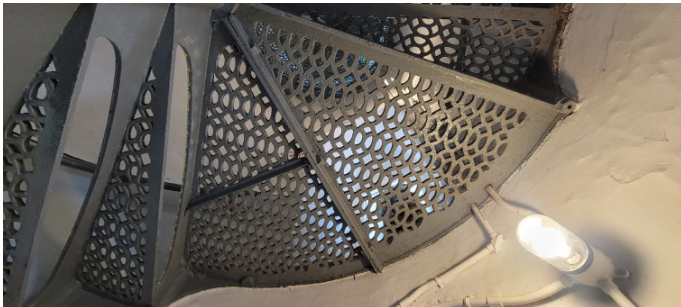
Figure 1D-258 Underside of lowest landing level (only two sections of the full circle, not a semi-circle like the other landings), note the left section is reinforced with a small metal angle at mid-length.
