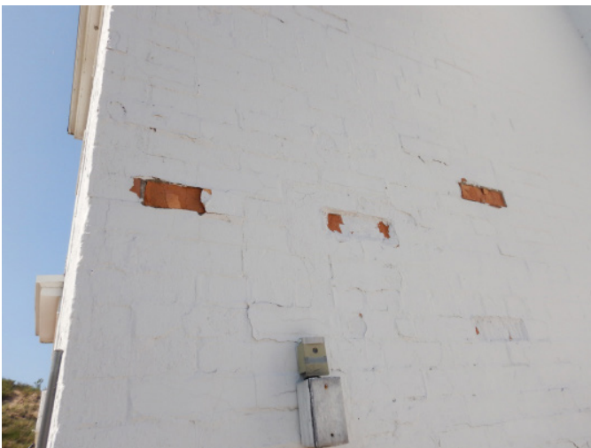
Figure 1D-65 Exposed red, spalled brick at east end of north façade where coating is missing.
