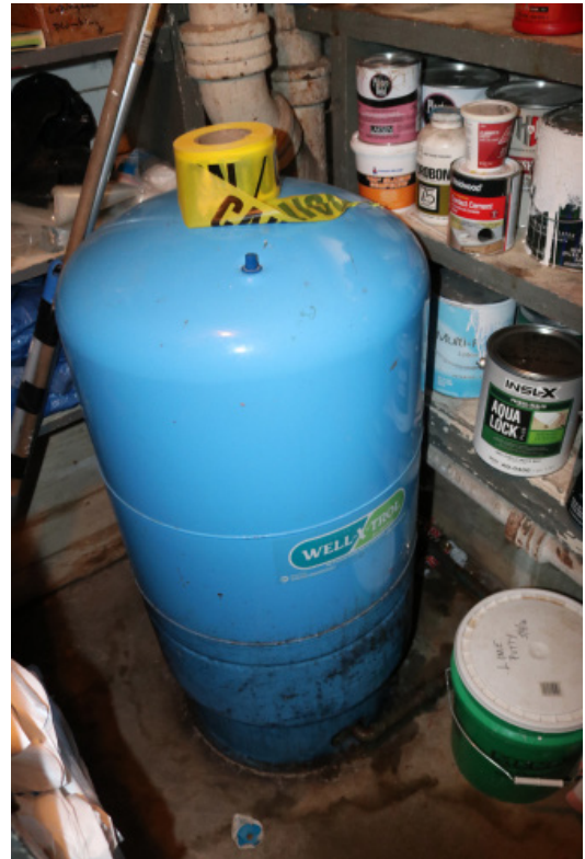
Figure 1D-196 Water well pressure tank located in the Basement.
