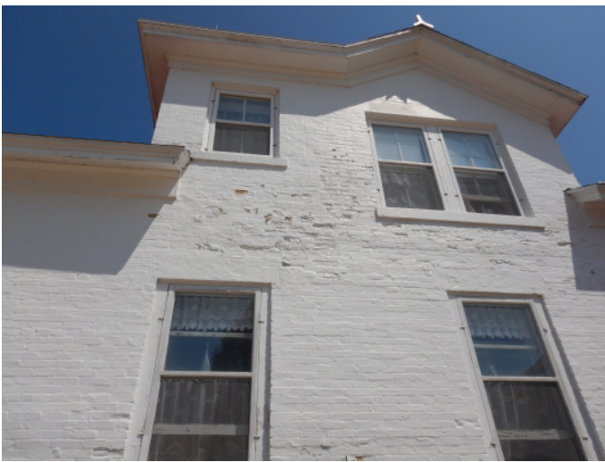
Figure 1D-71 Coating applied over spalled brick.
