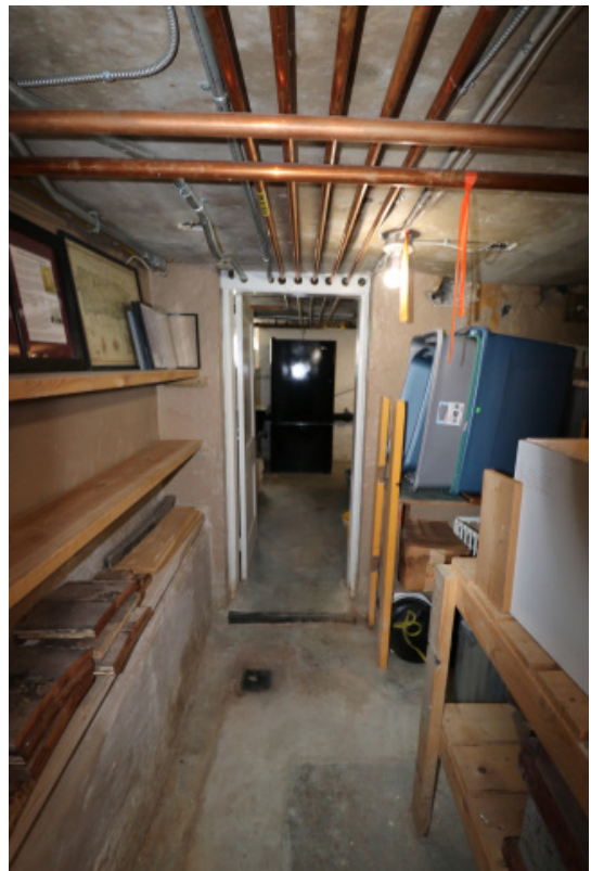
Figure 1D-197 Exposed copper water lines in the Basement.
