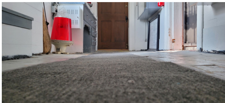
Figure 1D-228 Vertical displacement of paver floor.
