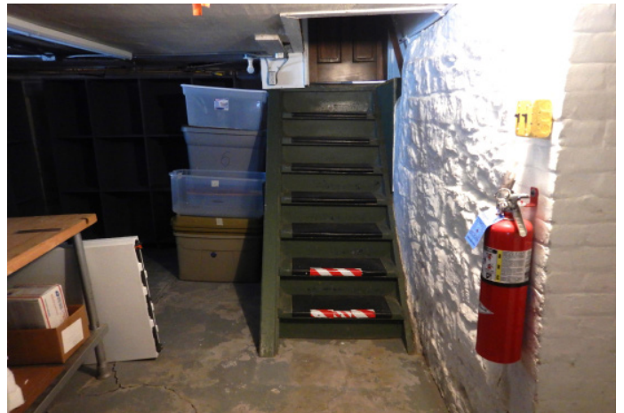
Figure 1D-39 Unlevel stair treads at basement stair in southwest quadrant of basement.
