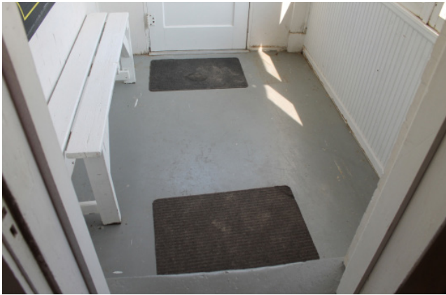
Figure 1D-49 Top surface of concrete slab in southeast corner of Keepers' Dwelling first floor level.
