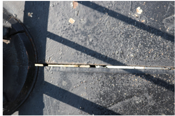
Figure 1D-296 Large gap between sections of the cast iron floor at the Watch Deck.
