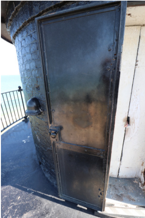
Figure 1D-290 Exterior steel plate door providing access from the Watch Room to the exterior Watch Deck.
