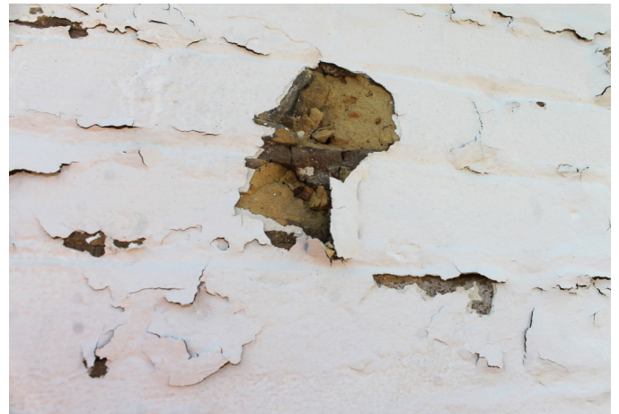
Figure 1D-67 Damaged buff colored brick behind coating which was peeling off of exterior surface of wall.
