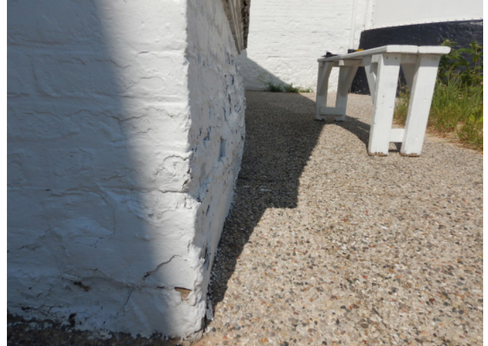
Figure 1D-77 Visibly displaced outward brick foundation wall of single-story projection on north facade.
