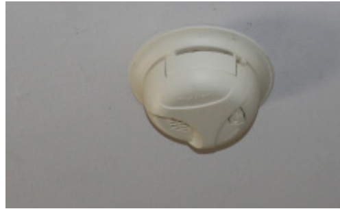
Figure 1D-220 Smoke detector/smoke alarm.
