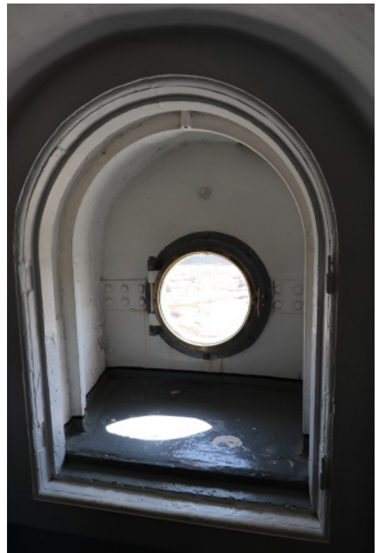
Figure 1D-283 Interior view of Porthole window and non-extant original arch top tower window.
