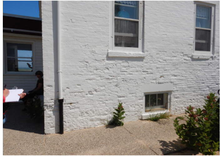
Figure 1D-70 Coating applied over spalled brick.
