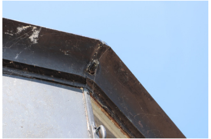
Figure 1D-305 Gutter drainage tube and cracking at cornice joint.
