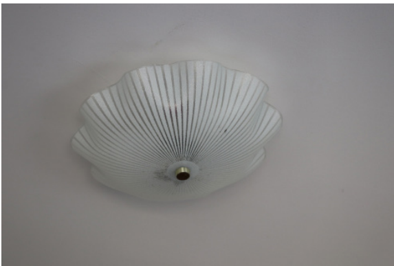
Figure 1D-215 Interior light fixture example.
