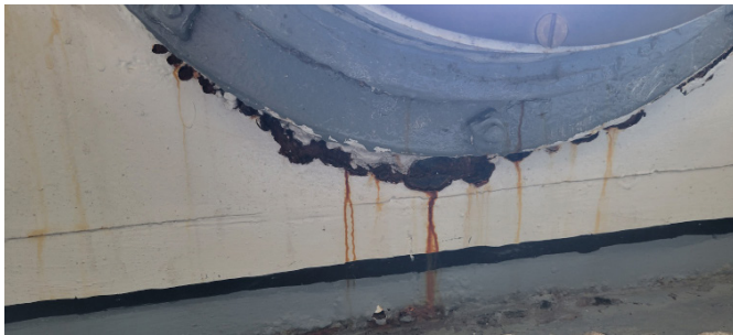
Figure 1D-251 Corrosion of steel plate below port hole window at watch room floor level.
