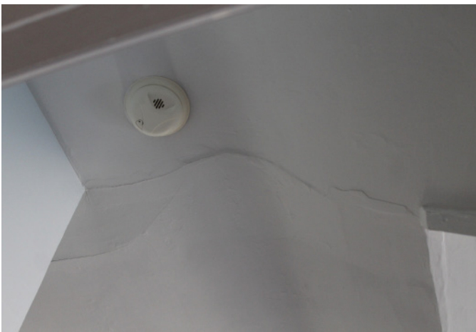
Figure 1D-56 Cracking between interior partition walls in ceiling.
