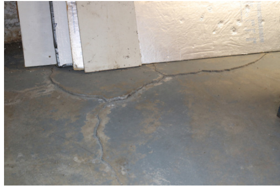
Figure 1D-192 Concrete floor slab cracking in the west part of the Basement.
