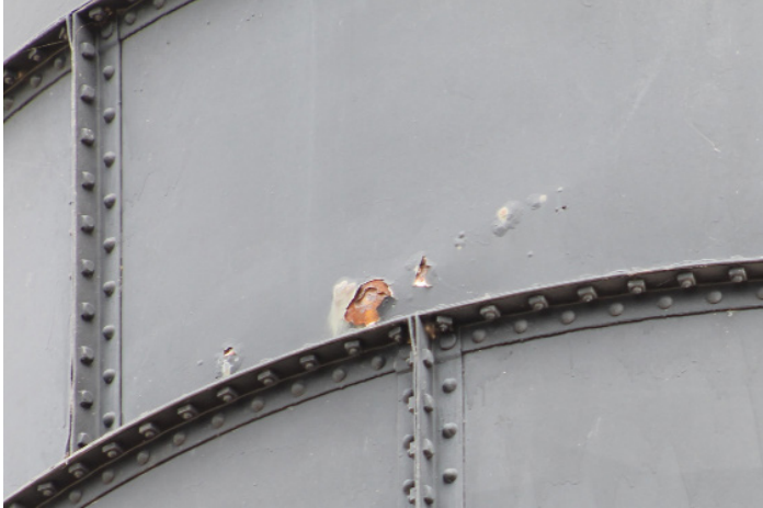
Figure 1D-267 Closer view of corrosion of metal cladding where coating is missing.
