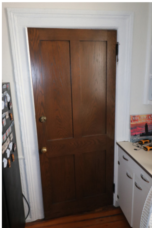
Figure 1D-171 Newer interior wood panel door in a Closet off of the first floor Gift Shop (former Kitchen).
