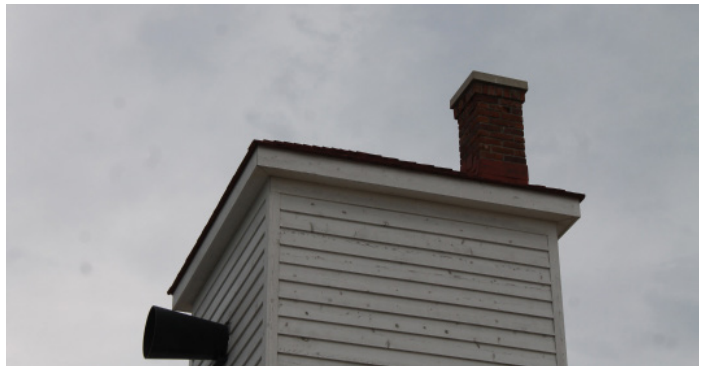
Figure 1D-339 Stepped sheet metal flashing at intersection of masonry chimney and roof of fog signal building.
