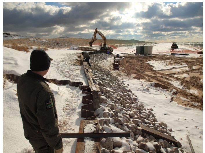
Figure 1B-104: Photo taken during construction of the south seawall extension in the winter of 2012 - 2013.
