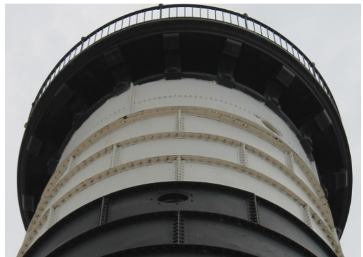
Figure 1D-272 Daylight observed through fastener holes in horizontal leg of angles where upper cladding meets lower cladding around perimeter of tower.
