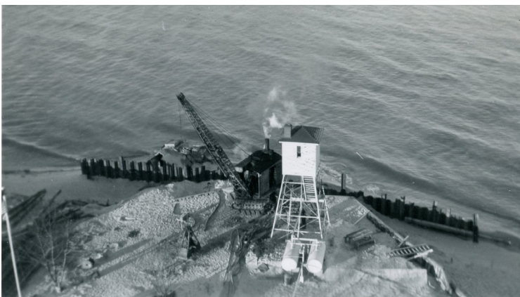
Figure 1B-59: Steel sheet piling being installed in the fall of 1943 to provide shoreline protection around the fog signal tower.
