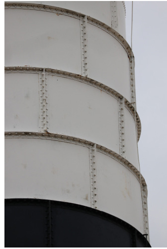
Figure 1D-277 Metal cladding on the Light Tower with "white" and "black" paint patterns.
