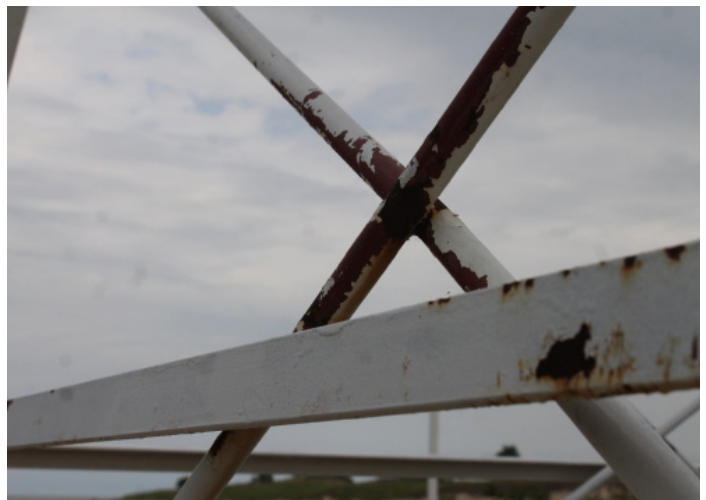
Figure 1D-335 Worn coatings and spotted corrosion of the steel tower frame.
