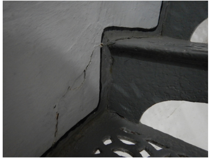
Figure 1D-248 Cracking in plaster at stair tread.
