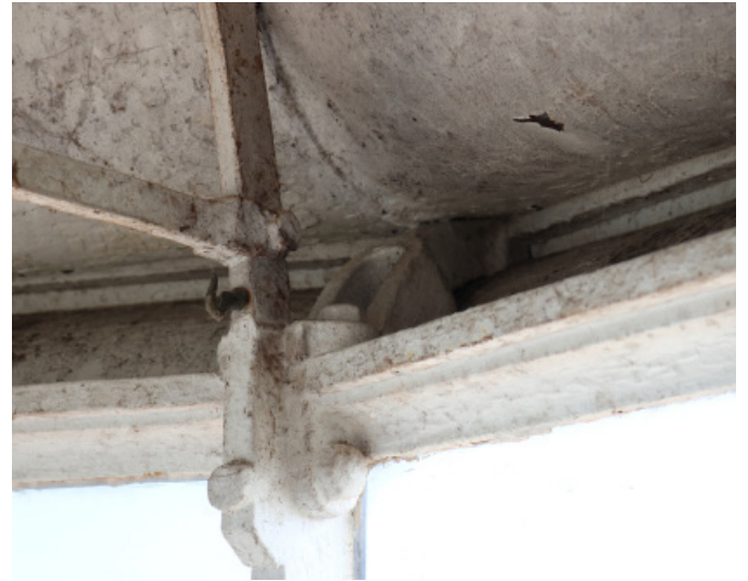
Figure 1D-327 Vertical mullion and upper frame around Lantern glass.
