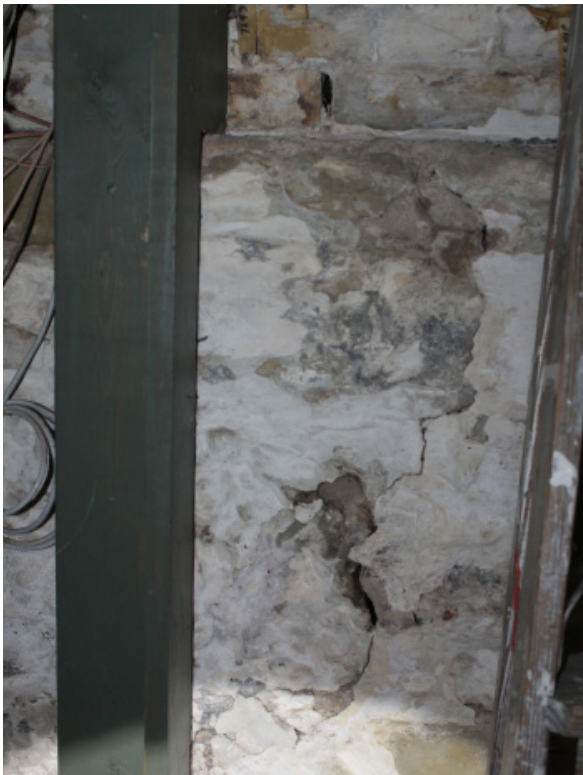
Figure 1D-40 Vertical cracking in upper courses of center stone masonry bearing wall.
