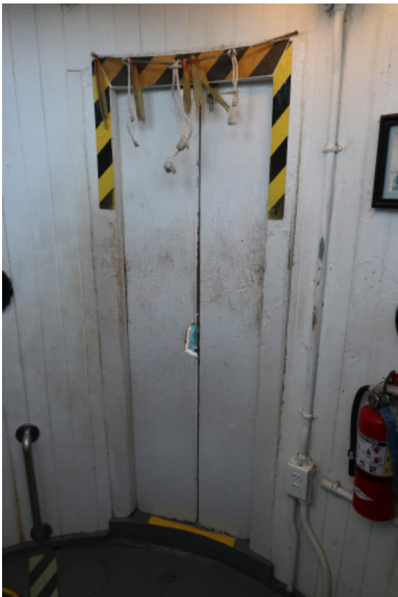
Figure 1D-294 Inner face of the pair of inner wood doors at the Watch Room.
