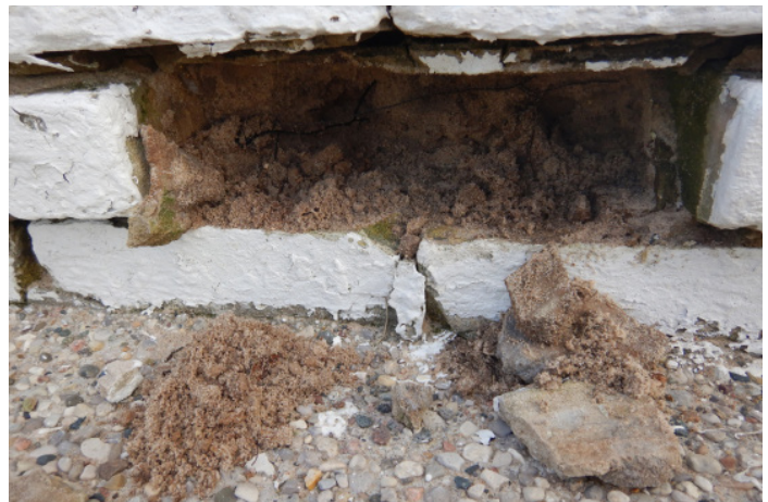
Figure 1D-79 Vegetation rooting in sand directly behind loose brick.
