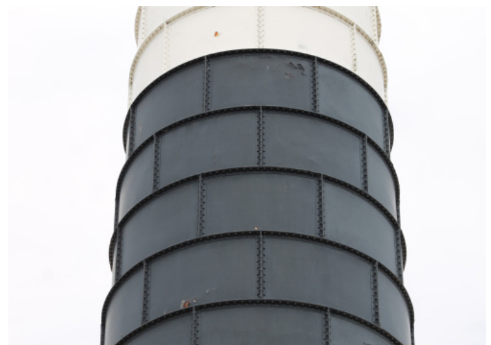
Figure 1D-266 Isolated areas of missing or peeling coating from metal cladding.
