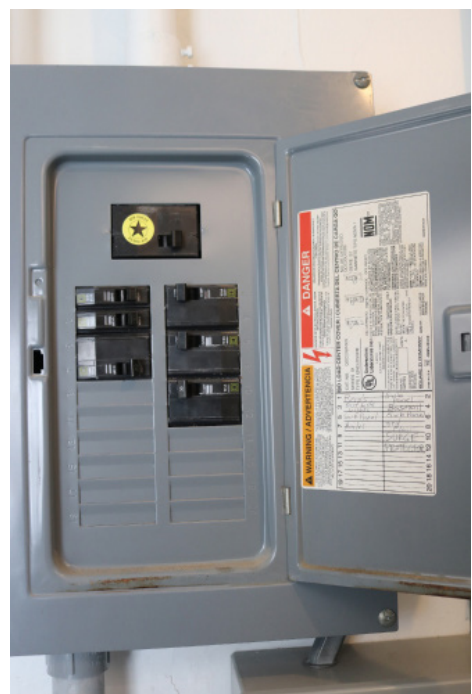
Figure 1D-242 Main 100 Amp electric panel.
