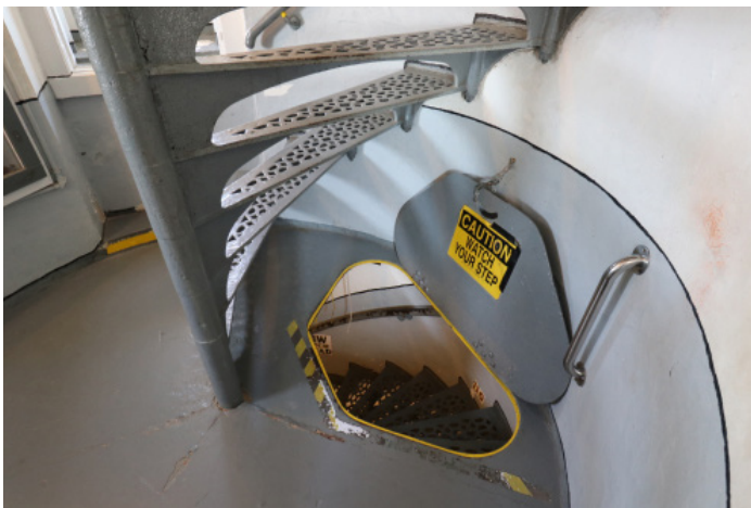
Figure 1D-312 Metal floor hatch at the fourth landing level. Note stainless steel grab bar.
