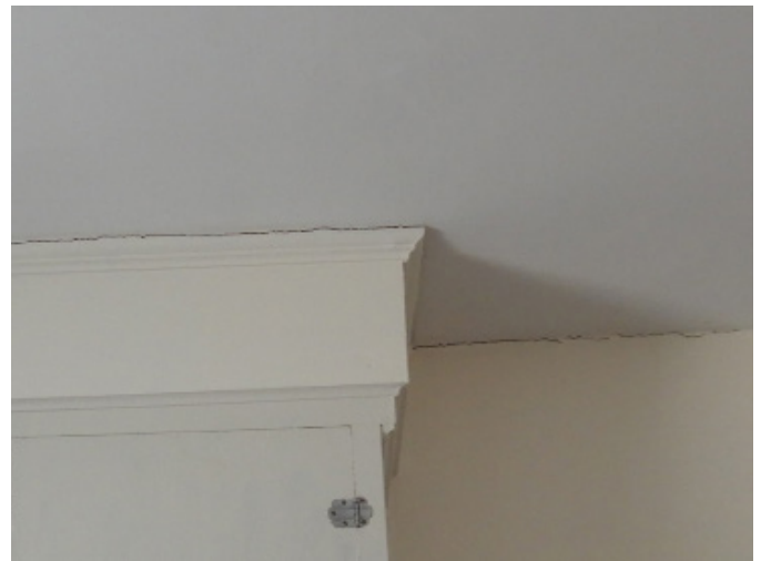
Figure 1D-52 Separation at ceiling and cupboard, and at ceiling and wall in first floor eastern kitchen space along east wall.
