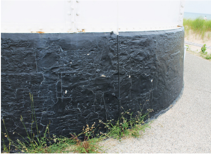
Figure 1D-263 Cracking in grid pattern through coating at base of tower; likely reflecting mortar joints of stone foundation.
