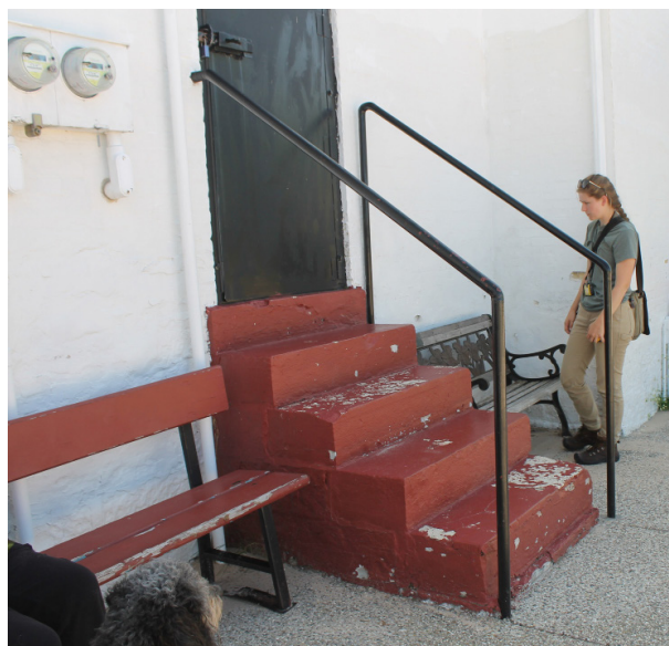
Figure 1D-222 Steps to west door of connector link; note top anchorage for rail differs each side of steps, north side is anchored to building wall and south side is anchored to steps.
