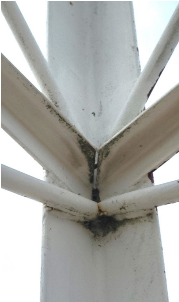
Figure 1D-336 Welded connections of steel bar cross bracing and third set of horizontal angle members located above grade at corner angle column of fog signal tower.
