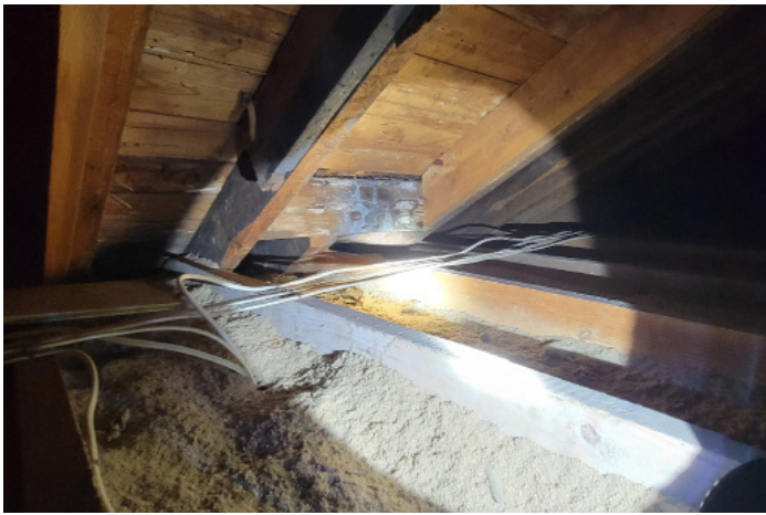
Figure 1D-62 Extensive water staining at south dormer framing at east half of roof.
