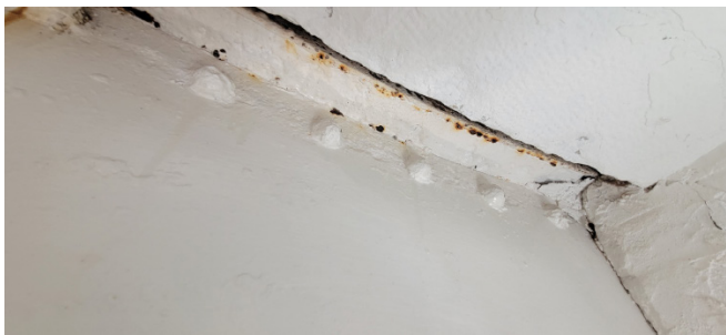
Figure 1D-252 Corrosion staining at window well at watch room floor level; note section loss of rivet heads on the right side of the photo.
