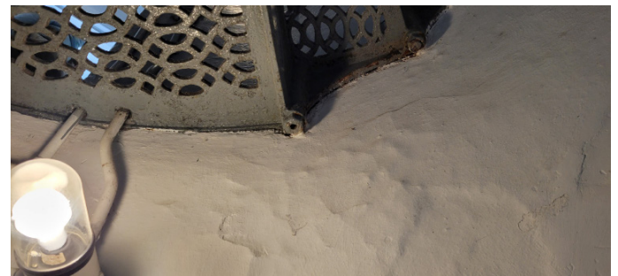
Figure 1D-249 Plaster distress below stairs; note bolt between treads does not extend down through assembly.
