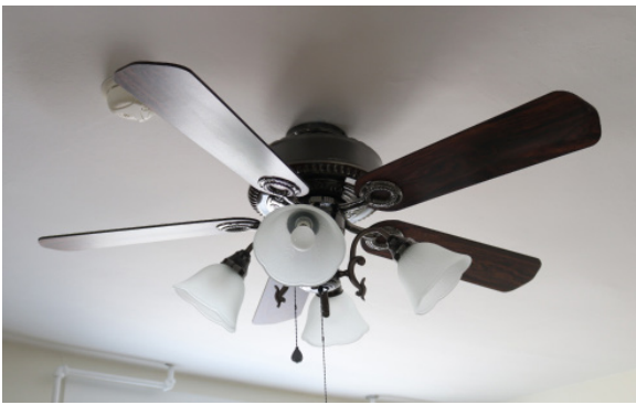
Figure 1D-213 Interior light fixture with fan.
