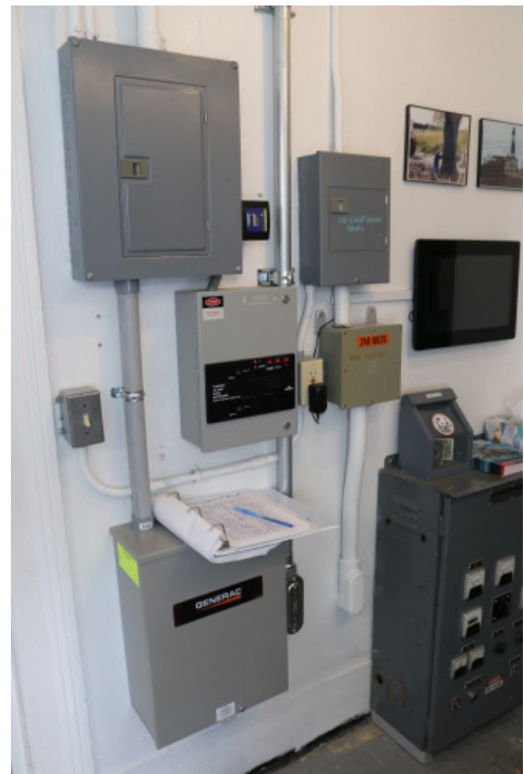
Figure 1D-241 Main electric panel and sub-panels on the west wall of the Passageway.
