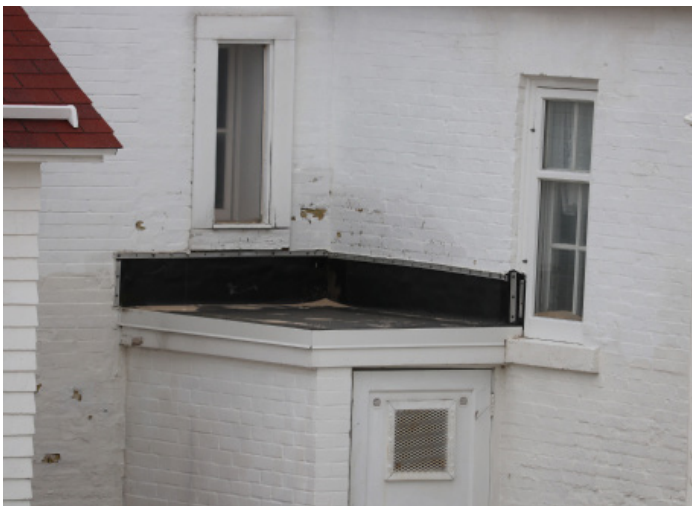
Figure 1D-86 EPDM roof on the Basement stair enclosure on the north side.
