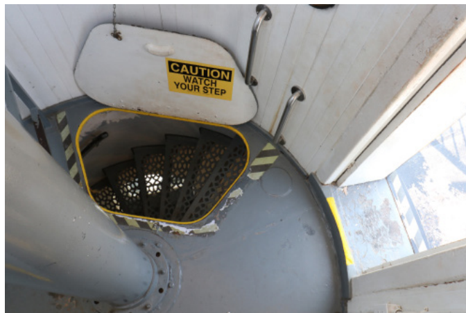
Figure 1D-314 Metal floor hatch at the Watch Room. Note stainless steel grab bars.
