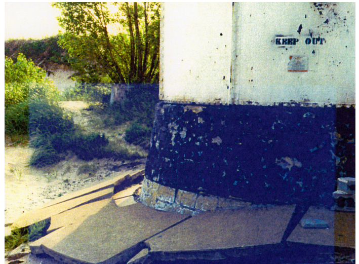
Figure 1C-28: Circa 1980s photo of the collapsed concrete walkway around the base of the tower.
