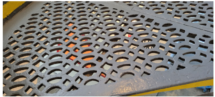
Figure 1D-260 Top surface of the same landing in Figure 1D-257, note reinforcing angle and cracking visible on top surface in lattice and turned down edge adjacent to other landing section.
