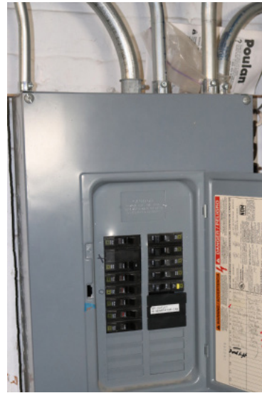
Figure 1D-210 Electric sub-panel located in the Basement.
