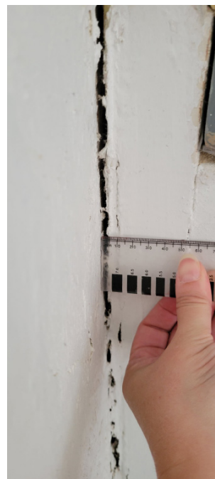
Figure 1D-226 Cracking present at north end of east wall at intersection of tower on interior.
