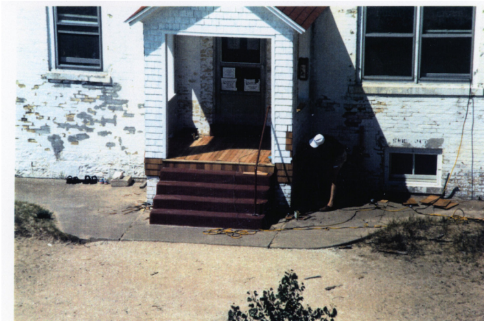
Figure 1B-97: Circa 1990s photo of SPLKA volunteers replacing the south porch flooring.
