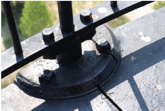
Figure 1D-297 Cracked railing base plate.
