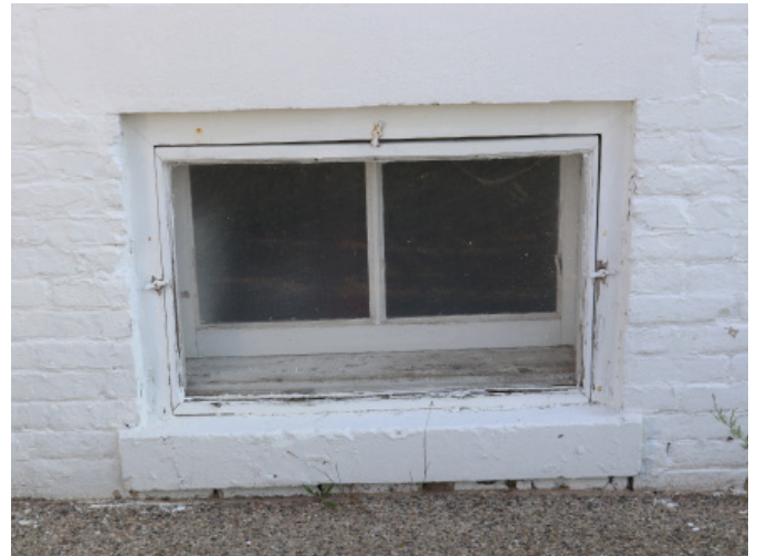
Figure 1D-98 Basement window and deteriorated storm sash on the north elevation.
